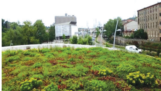
DRY WEATHER INSPECTION OF PWD'S VENICE ISLAND PUMPHOUSE GREEN ROOF [LOOKING NORTH]
