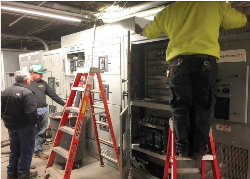
REPLACEMENT OF OIT’S SUB-BASEMENT ELECTRICAL GEAR AND TRANSFORMER THAT SUPPORTS ELECTRICAL POWER FOR OIT’S DATA CENTER, THE CENTRAL HUB OF THE CITY’S NETWORK AND MISSION CRITICAL APPLICATIONS.
