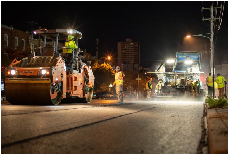
STEAM RISES OFF FRESH ASPHALT UNDER THE GLOW OF WORK LIGHTS AS PAVING CREW WORKERS OPERATE HEAVY MACHINERY DURING OVERNIGHT STREET RESURFACING ON WASHINGTON AVENUE.
