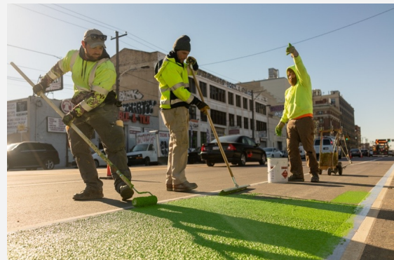
WORKERS ADD BRIGHT GREEN PAINT TO BIKE LANES ON THE NEWLY REPAVED WASHINGTON AVENUE.
