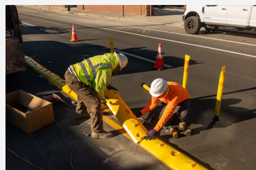
WORKERS INSTALL BRIGHT YELLOW MODULAR CURBS AS PART OF A HARDENED CENTERLINE ON WASHINGTON AVENUE.
