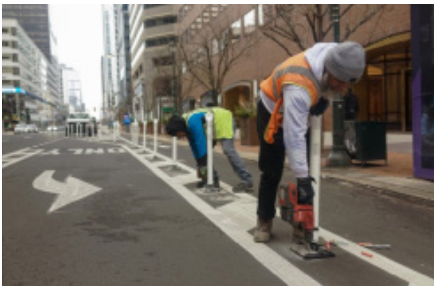
STREETS DEPARTMENT WORKERS INSTALL FLEX POSTS FOR THE PARKING PROTECTED BIKE LANE ON THE NEWLY REPAVED MARKET STREET NEAR 18TH STREET.
