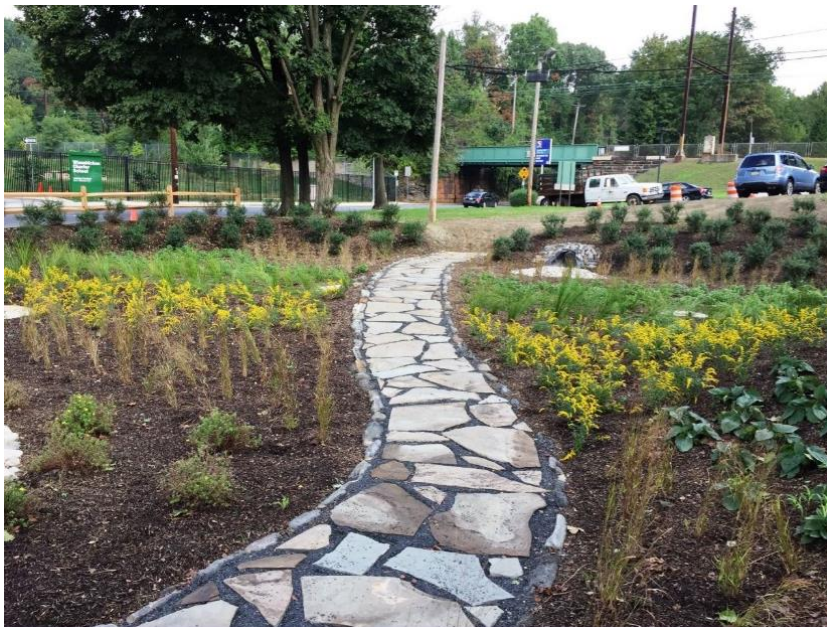
A thriving rain garden, constructed by the Philadelphia Water Department in 2016, drains over 38,000 sq. ft. of stormwater runoff in Germantown.
