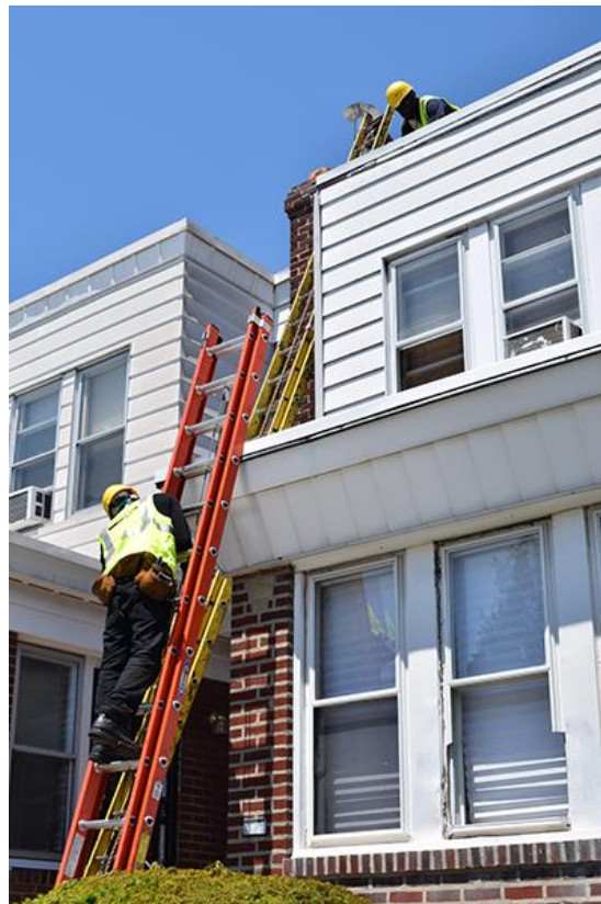
Workers providing roof repairs as part of the Basic Systems Repair Program.
