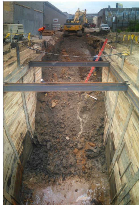
A large trench is excavated along Laurel Street for a box sewer, part of the Northern Liberties Storm Flood Relief project (NLSFR) to double the capacity of the system it is replacing.
